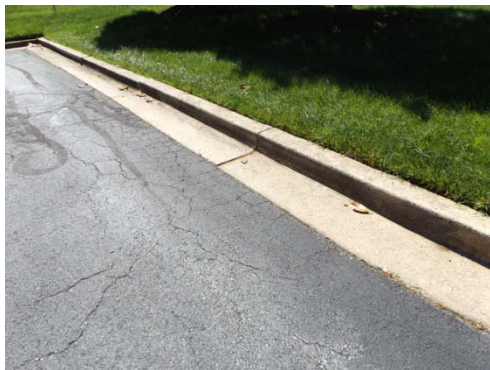
Photo 1 - Cracking & alligating, typical
