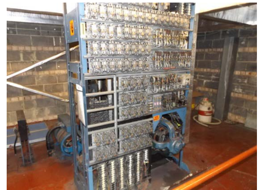
Photo 21 - Elevator control relays
