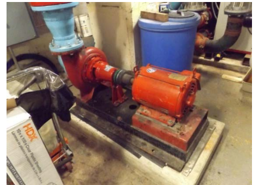
Photo 19 - Typical circulation pump
